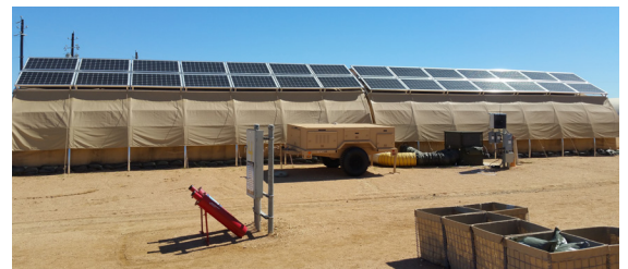
Lackland AFB, Texas. At expeditionary microgrid system at Lackland AFB, monocrystalline silicon solar panels are placed on top of each tent for energy production while a trailer (center) holds the hardware, software, and lithium-ion batteries that form the smart grid. U.S. Air Force Photo by Donna Lindner. February 2, 2016.
