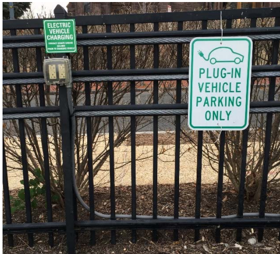
Level 1 charging receptacles are available for use by U.S. Senate employees (U.S. DOE Photo)
