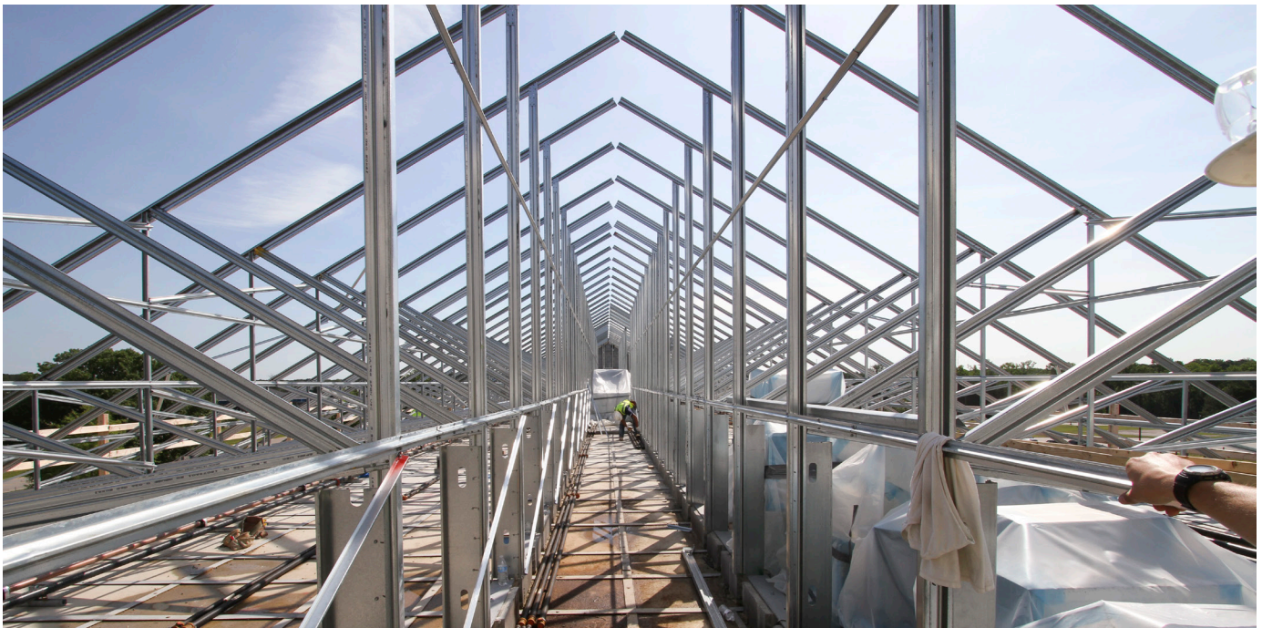
Figure 7: Contractors upgrade a 50-year-old facility at Fort Lee, Virginia with modern technology and force protection features.
