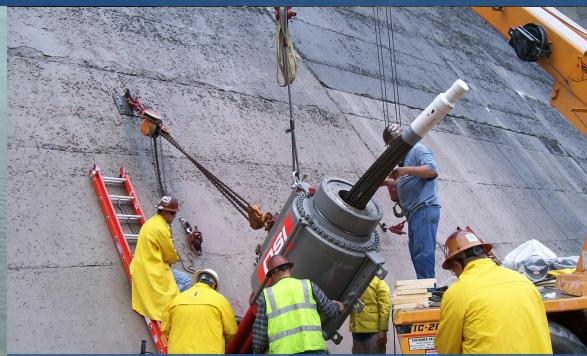
Construction crews place steel cables anchoring the Bluestone Dam into the bedrock, increasing the strength of the dam.
