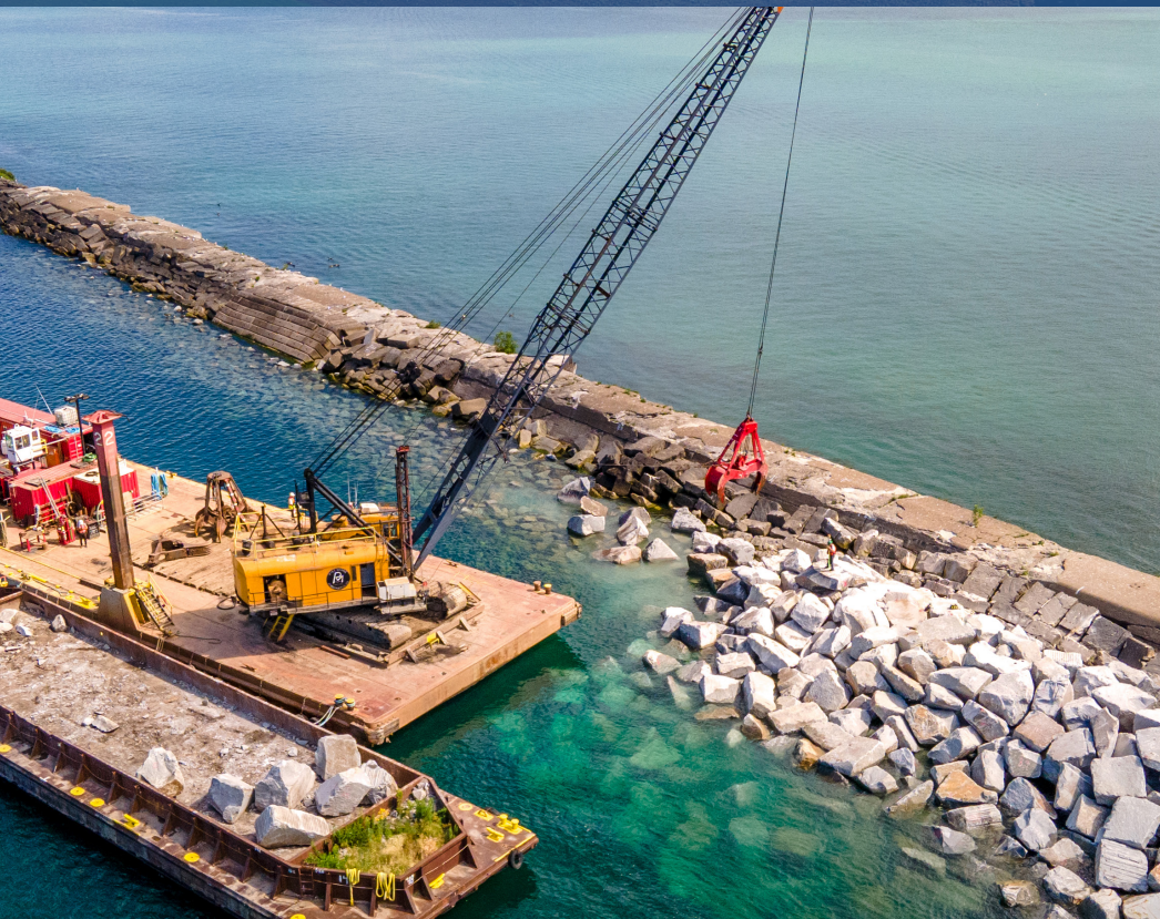
Construction and repairs to the 10,200-foot south breakwater that protects the Buffalo Harbor and nearby dredged sediment confined disposal facilities from deep water wave and ice action.
